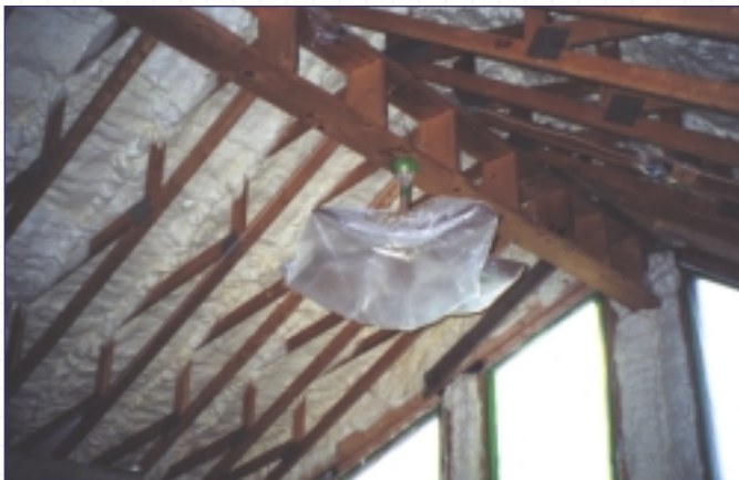
Icynene® is sprayed to a depth of 5 1/2 inches and adheres directly to the roof deck.
