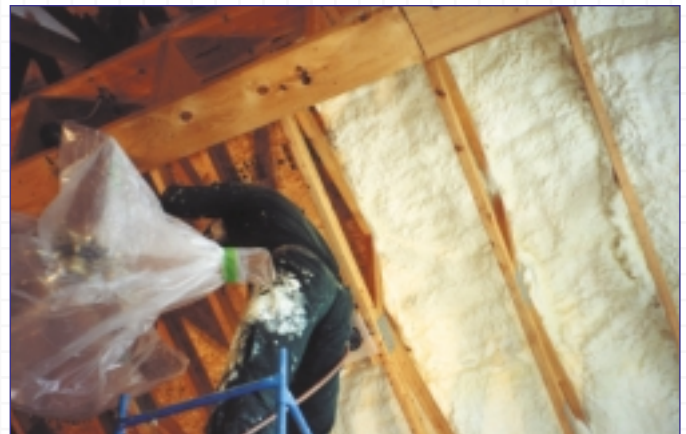
Icynene® is sprayed directly on to the roof deck. There are no air vent channels.
