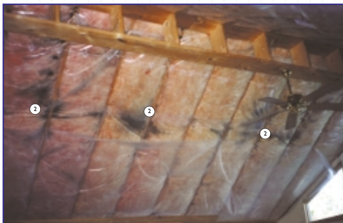
(2) Hot humid interior air had leaked past the poly, through the batt insulation, and come into contact with the cold air in the venting, thus causing condensation and mold.
